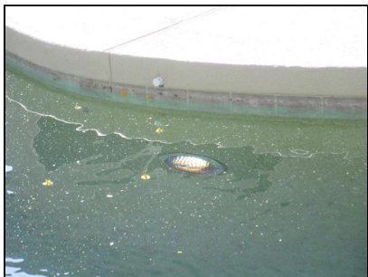
15.8 Item 1(Picture) Pool light functional
