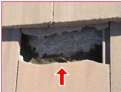
4.0 Item 4(Picture) Broken tile and damaged/exposed underlayment
