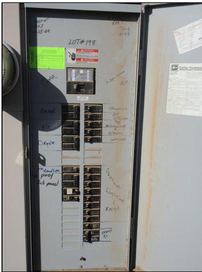
6.2 Item 1(Picture) Labeled Dead-front panel
