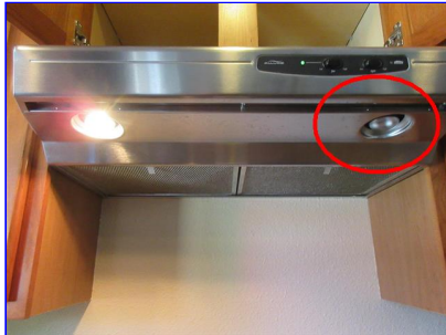
11.7 Item 1(Picture) Recommend replacing bulb
