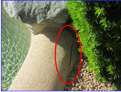
15.1 Item 1(Picture) Cracked coping
