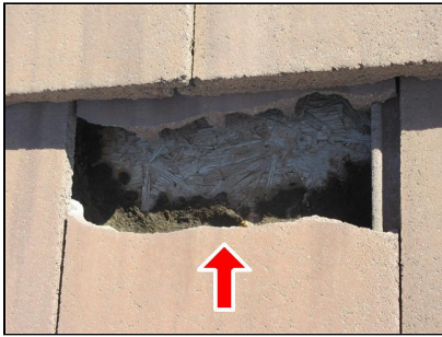
4.0 Item 4(Picture) Broken tile and damaged/exposed underlayment
