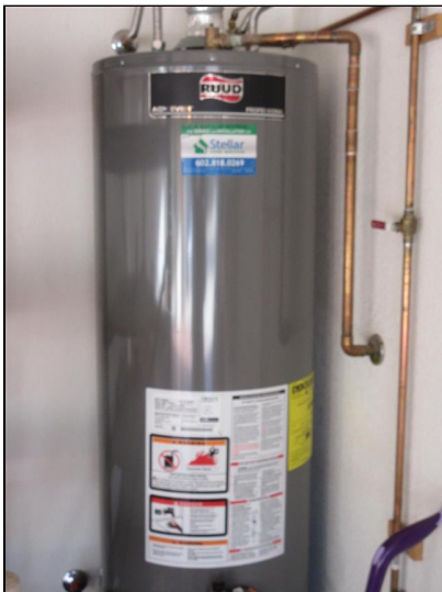
5.5 Item 1(Picture) RUUD Water Heater
