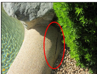
15.1 Item 1(Picture) Cracked coping
