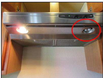
11.7 Item 1(Picture) Recommend replacing bulb
