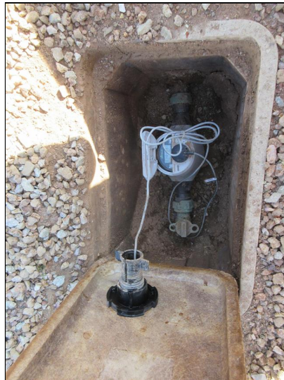
5.1 Item 2(Picture) Main water meter southeast front corner of home
