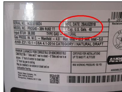
5.5 Item 3(Picture) Water heater MFG 2008 and is 40 Gals
